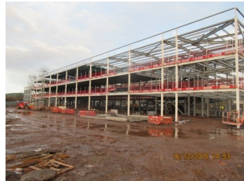
Photograph 8 – West elevation showing the completed structural steelwork from Grid A to U
