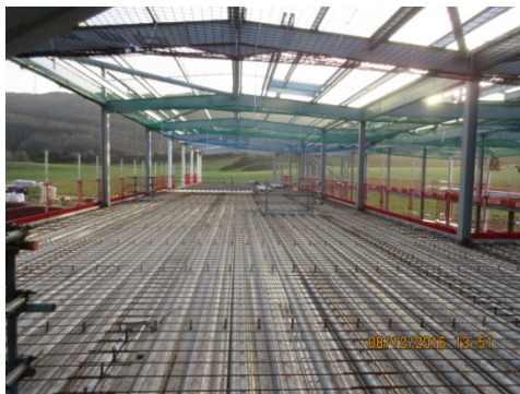
Photograph 3 Reinforcing installed to 1st and 2nd floor up to grid point M
