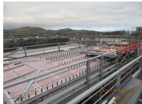
Photograph 2 Roofing contractors progressed onto working on roof grid lines E to G
